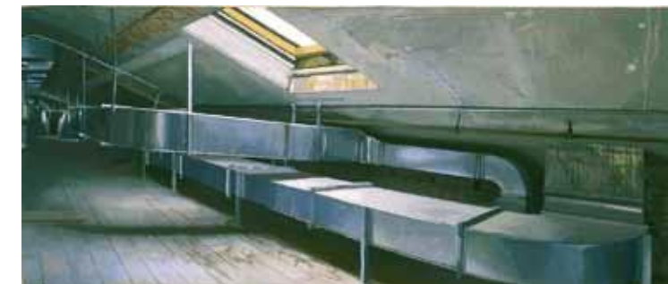
Left, Snug Harbor, Metal Ductwork in G Attic , 2001, oil on canvas, four panels, 16 by 168 inches overall. Iannan Foundation, Santa Fe.
